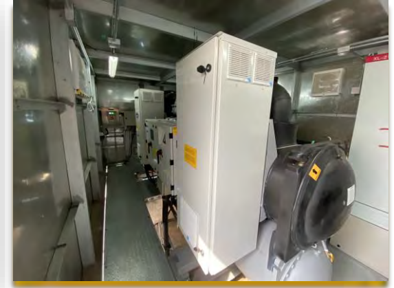
Chiller control panel
