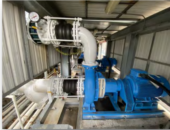
New chiller water pumps
