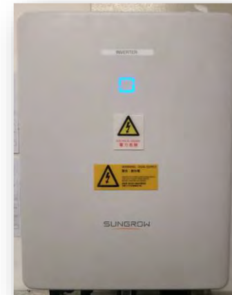
New installed inverter
