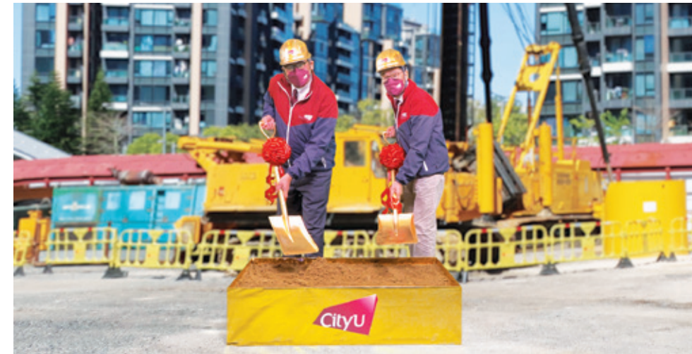
Construction started in March 2022 for the CityU Student Hostel project at Whitehead, Ma On Shan. 城大於馬鞍山白石的學生宿舍項目於2022年3月正式動土。
