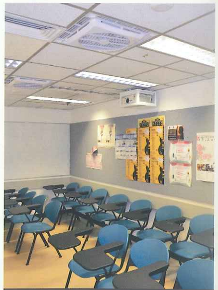
Installing fans in classrooms not only cut back on air conditioning, but also improve indoor ventilation and air quality.
