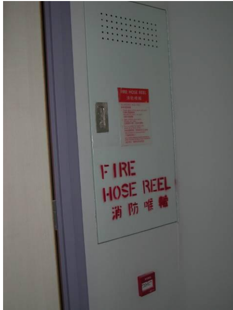
Fire hose reel
