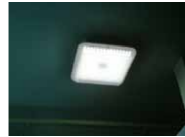
LED luminaires with sensors inside hall toilets: replace damaged fluorescence tubes with energy-efficient luminaries.
