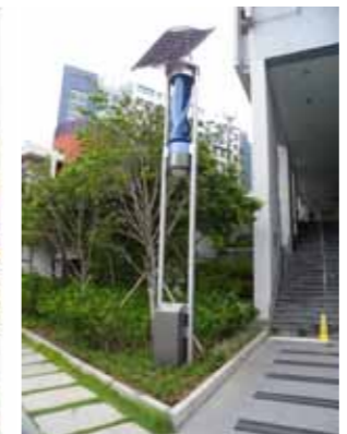
Solar-and-wind light towers: create adequate lighting in the areas by harnessing natural resources without consuming electricity
