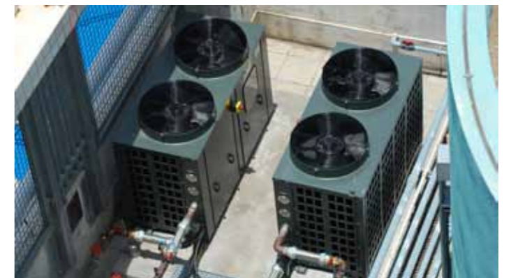
Heat Pump Project: deliver stable hot water supply in an energy-efficient manner.
