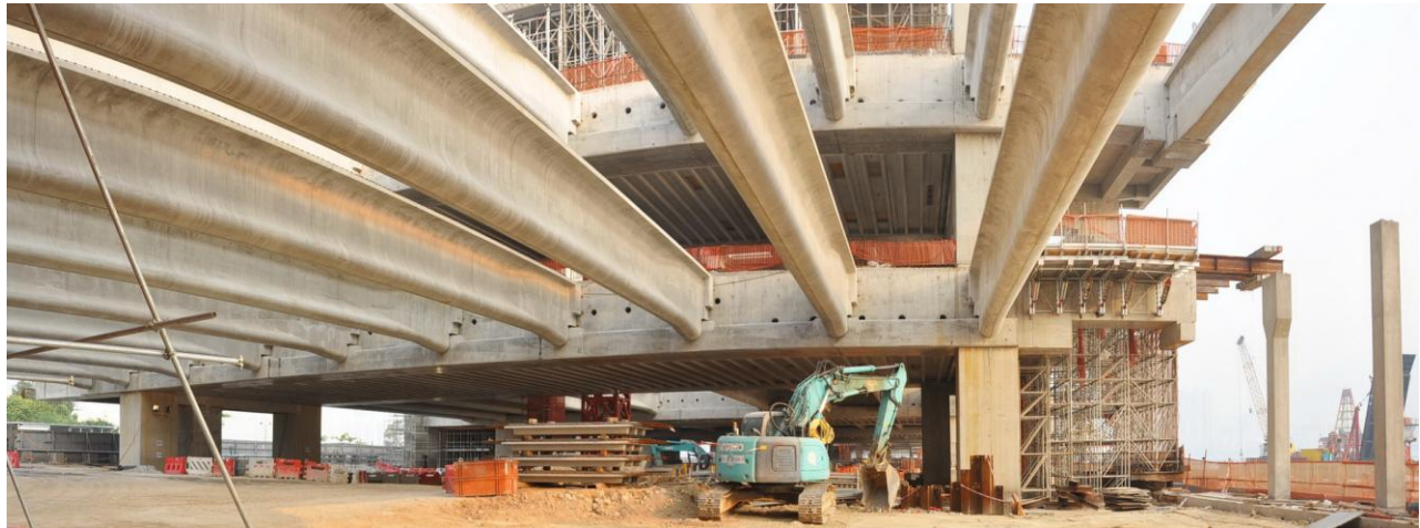
Photo description - The gigantic structure of the Cruise Terminal using large amount of precast long-span elements
